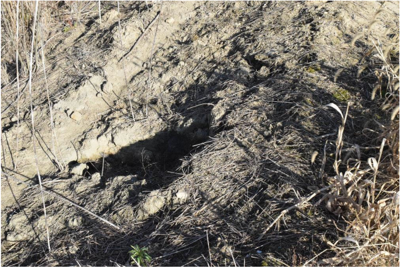
West side downstream slope – repair depressions and erosion
