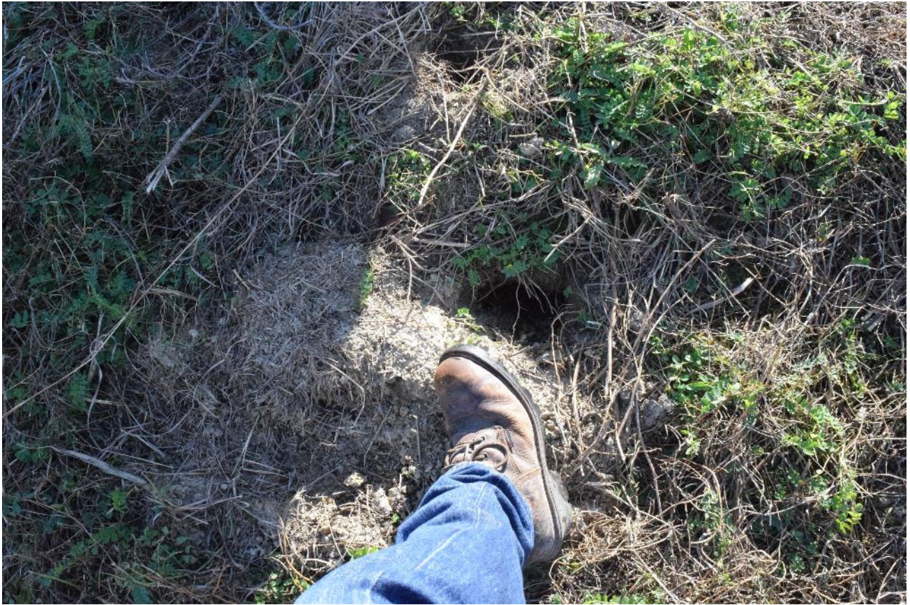
West side downstream slope animal burrow – fill
