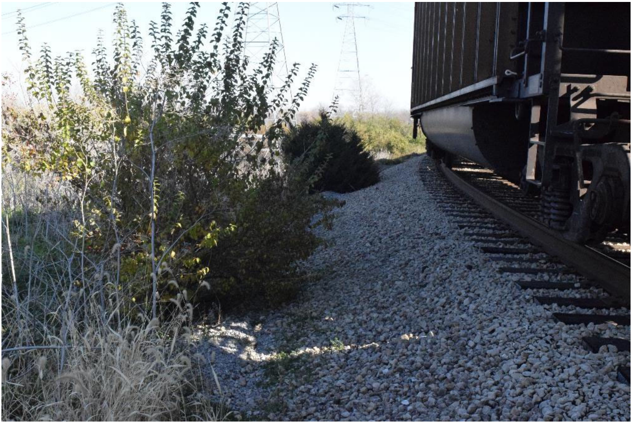
North side crest/downstream slope – remove trees
