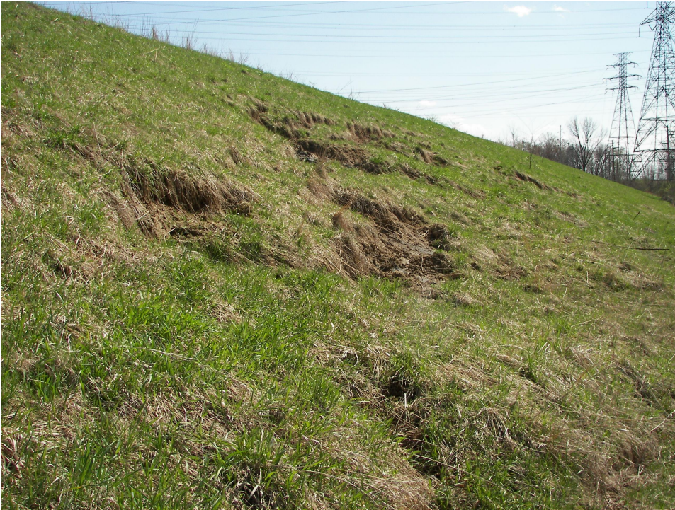
Figure E.1: Photo of 2009 Surficial Movement
