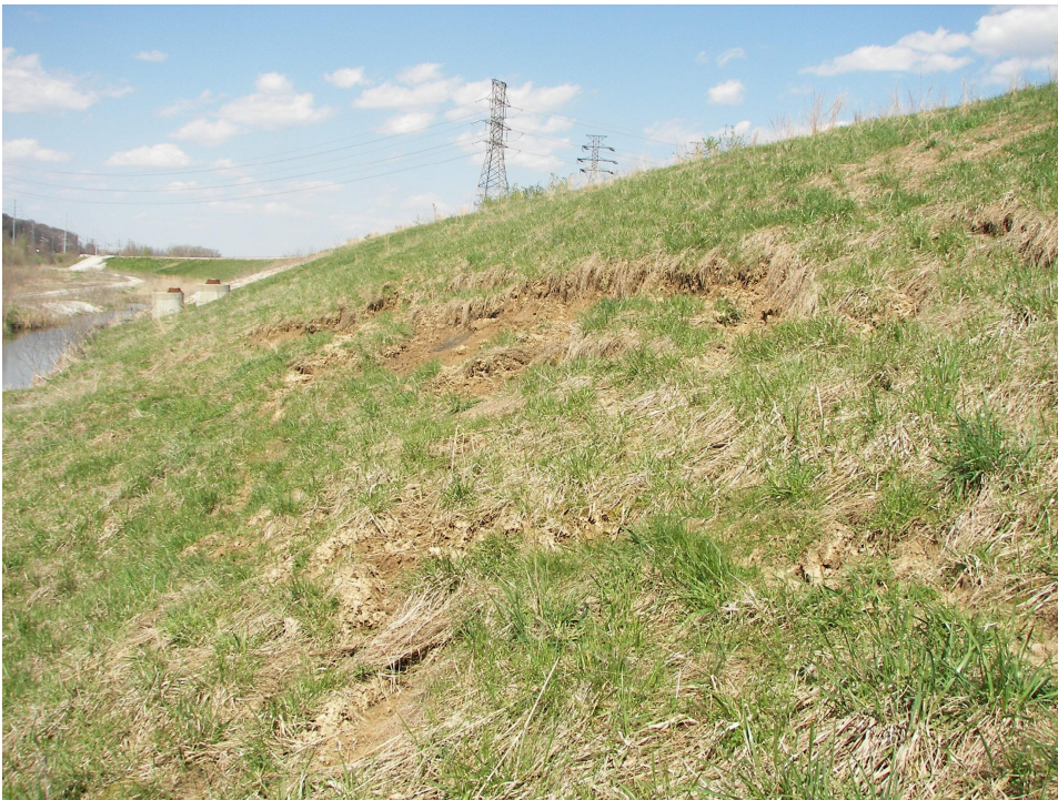
Figure E.2: Photo of 2009 Surficial Movement
