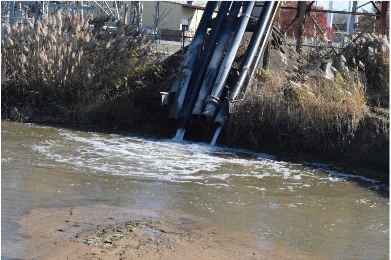
Outlet from plant
